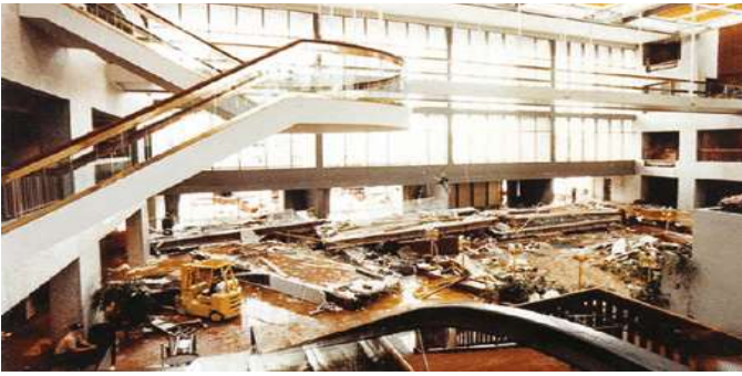
Figure 4 Situation at Hyatt regency Kansas City Walkways
