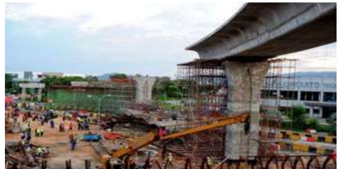
Figure 3 The collapsed ramp
