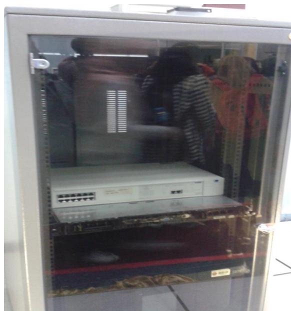
RACK SERVER AND TOWER SERVER
