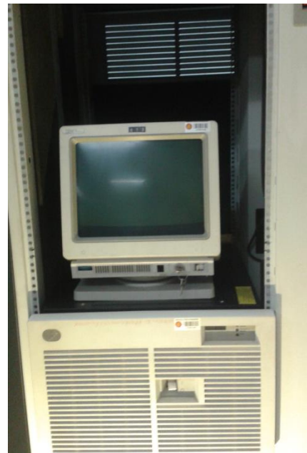
MAINFRAME MAIN SYSTEM POWER model: IBM 9309 2
