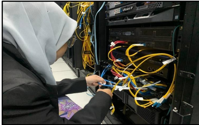
Figure 2.21 Cable Labelling on Switch
